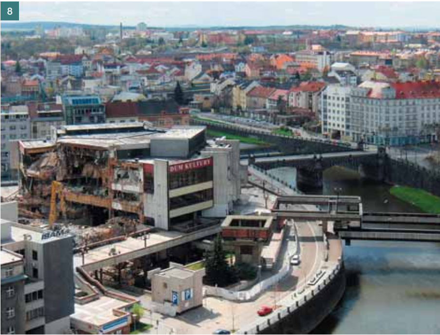
Obr. 8 Demolice kulturního domu ROH v Plzni, Miroslav Hrubec, 1986 (foto: Alexandra Hoffmannová) ■ Fig. 8 Demolition of the House of Culture of the Trade Unions in Pilsen, Miroslav Hrubec, 1986 (photo: Alexandra Hoffmannová)
