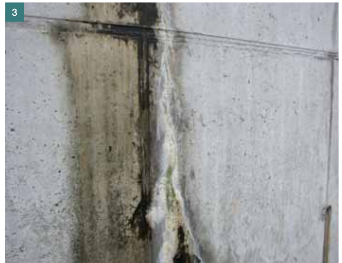
Obr. 3 Výluz z betonu po karbonataci | Fig. 3 Leach from the concrete after carbonation
