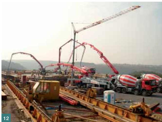
Obr. 12 Standardní sestava pro betonáž, dvojice čerpadel s domíchávači ■ Fig. 12 Standard arrangement for concreting, two concrete pumps and truck mixers
