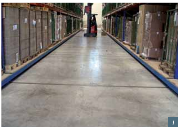
Fig. 4 Test core in the area of the crack
