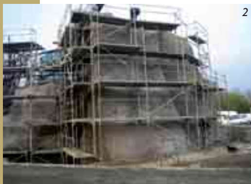
Fig. 2 Final modelling of the surface and setting of steel bearing spacers for the assembly of holds
