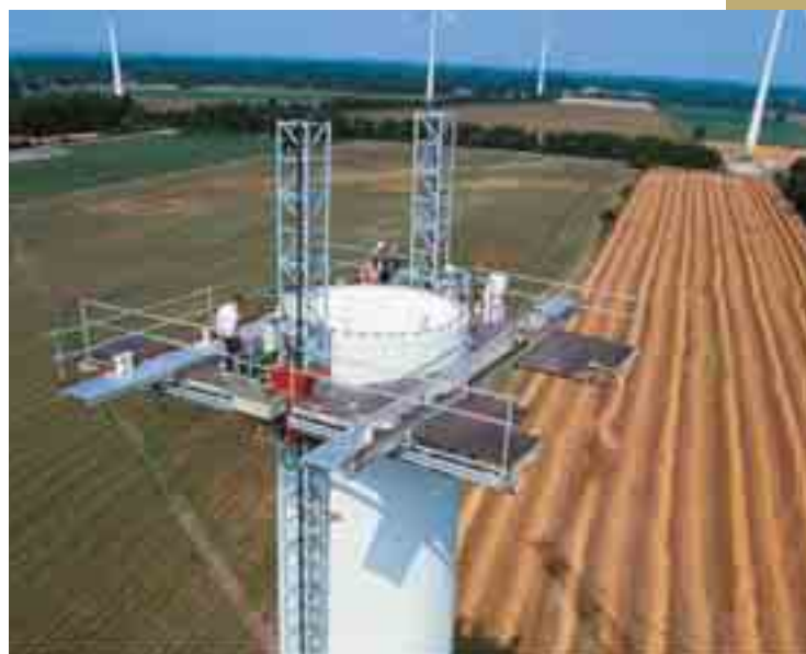
Fig. 2 Two HEK MSHF mast climbing work platforms connected using specially engineered bridges
