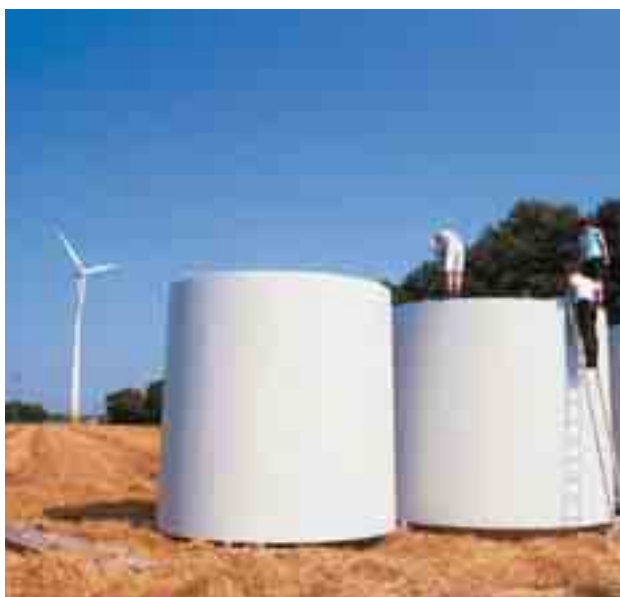
Fig. 1 3,8m high precast concrete elements of wind farm tower prepared for assembling
