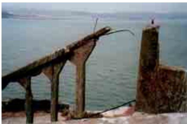
Fig. 4 Corrosion of a concrete guardrail: declination of a concrete structure in a double sense
