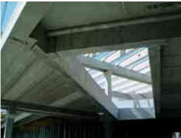
Fig. 12 Atypical composition of the floor structure with an opening for the escalator placement
