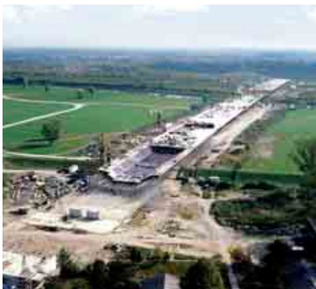
Obr. 34 Pohled na rozestavěný most Vlasti Fig. 34 A view of the Homeland bridge under construction
