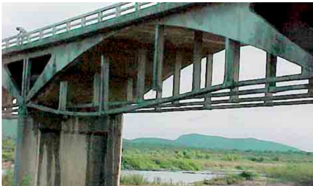
Fig. 4 Aspect of bent tie concrete and pulled down hung elements
