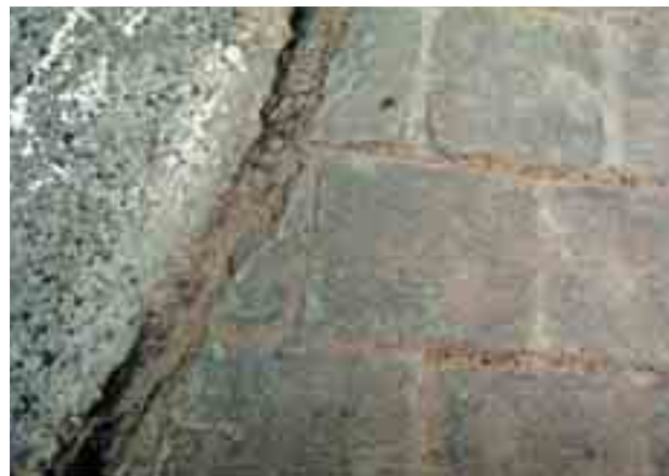
Fig. 5 Borderline between unrepaired and repaired imitated concrete flagstones
