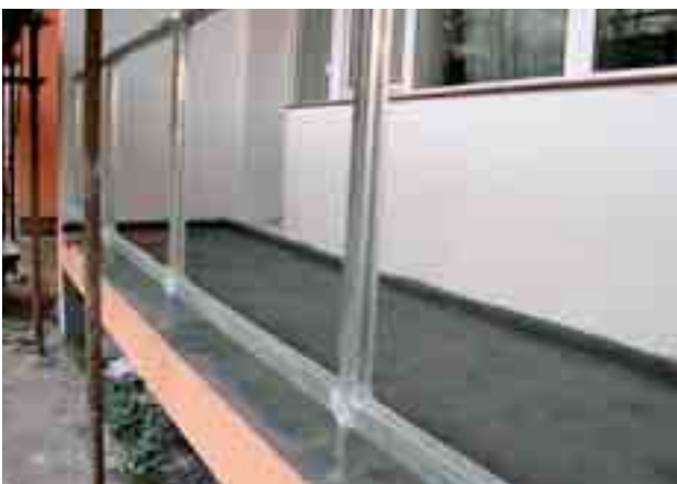
Fig. 7 View of loggia painted by crystalline material during reconstruction of the panel block of flats in Tobruč str. in Prague 6
