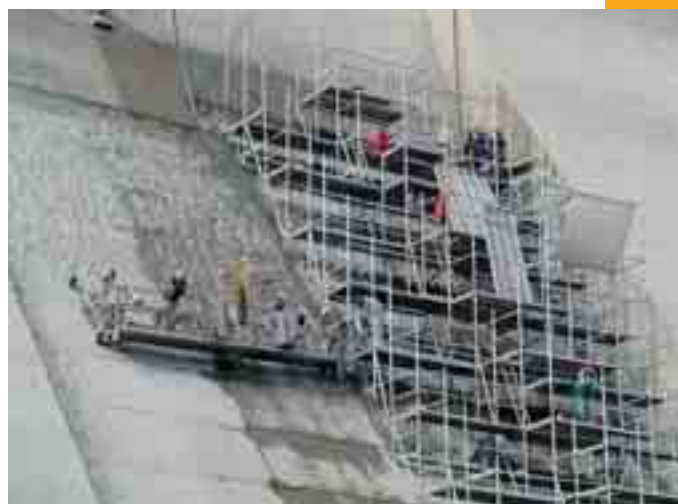
Fig. 4 Securing access to the downstream face by means of a combination of a stationary scaffolding and a mobile footbridge
