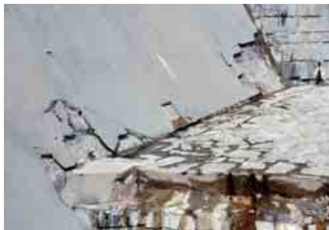
Fig. 8 Damage of the repaired concrete surface spillway in connection with a cascade
