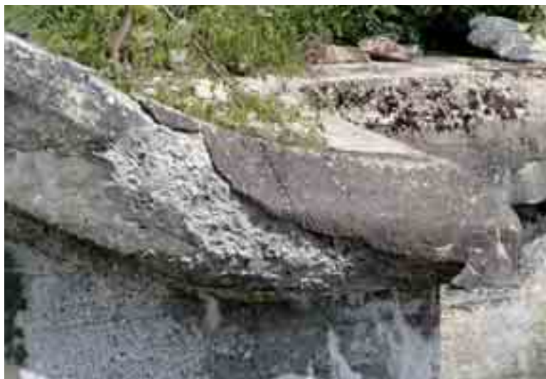
Fig. 1 Damage to the concrete of the end of the external wall of the stilling basin
