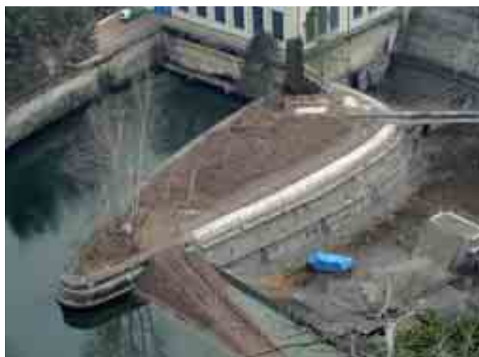
Fig. 3 View of the drained stilling basin during the repair of the separating structure
