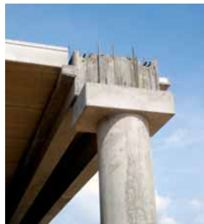
Fig. 6 Detail of the placement of a girder and a floor panel in a continuous cantilever
