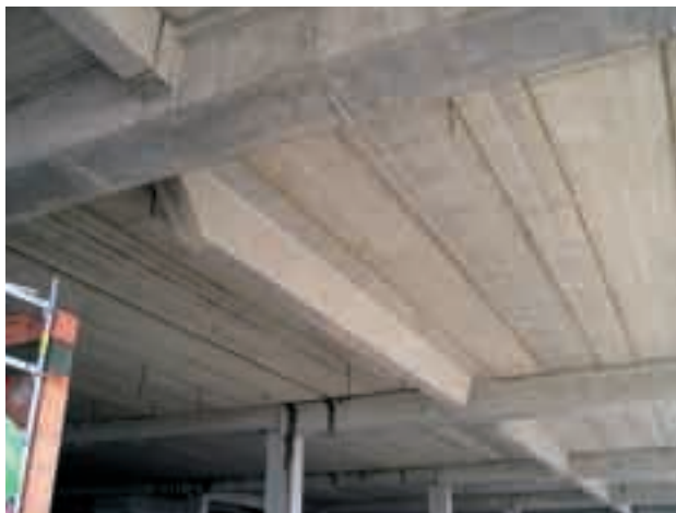
Fig. 11 Floor beam with openings for running through suspensions of the steel structure
