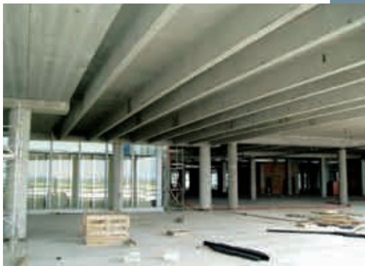
Obr. 16 Fischerova hala se stropními panely TT Fig. 16 Fischer's hall with TT ceiling panels
