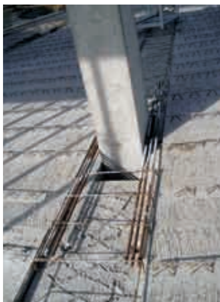
Fig. 7 Twin cross-beam with additionally laid upper reinforcement above the support. The bearing area of the additionally laid concrete with protruding reinforcement and roughened surface
