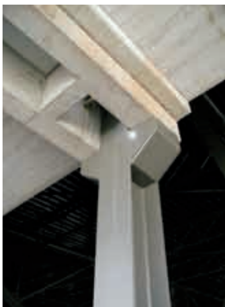
Fig. 5 Twin beam with an opening for wiring and piping placed on a steel column carrying the roof cover of the hall
