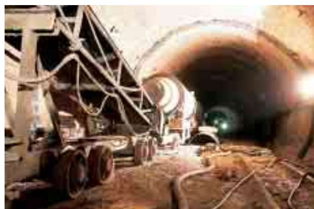
Fig. 2 The conveying system for fresh concrete transport with the application of a secondary jamb
