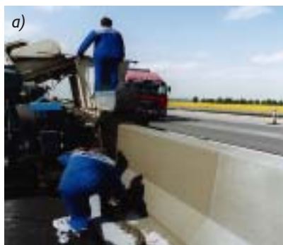
Fig. 3 Minipower SGME in building monolithic concrete safety fences 1.1 m high – a) front view, b) rear view
