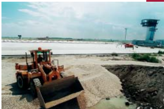
Fig. 5 Placement of cement concrete cover at the international airport MRS in Bratislava
