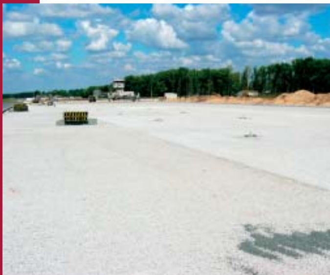
Fig. 1 A layer of gap-graded concrete in the AB Čáslav; formwork preparation in the background
