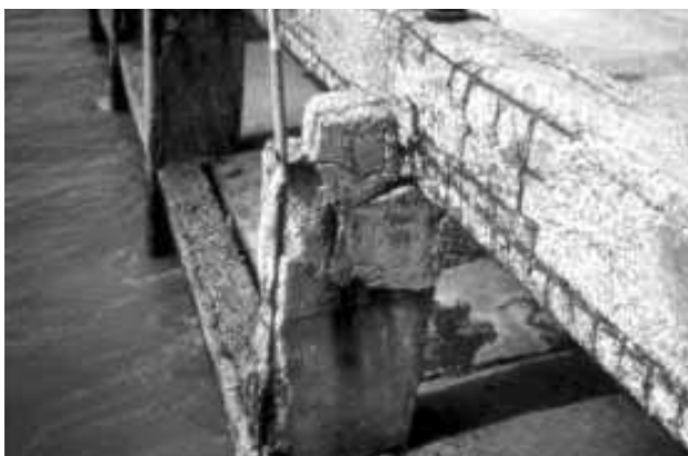
Fig. 4 Reinforced concrete jetty in the Arabian Gulf exhibiting extensive chloride induced corrosion damage
