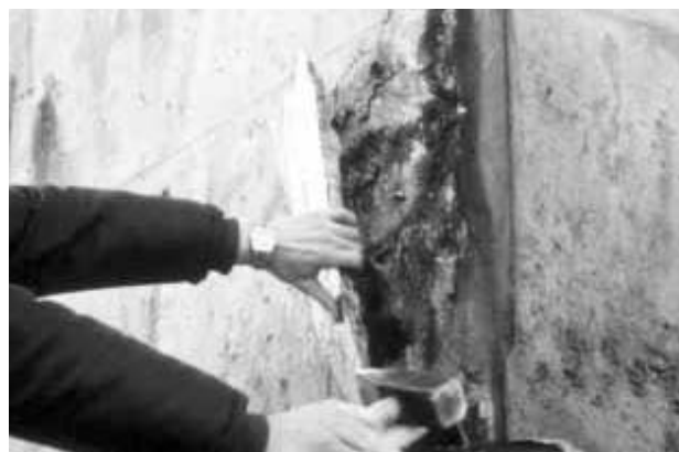
Fig. 5 Bridge piers exposed for 18 years to a temperate marine environment
