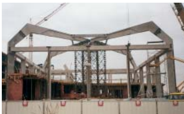
Fig. 18 Load-bearing RC structure supported at the centre with a steel framed structure before making it monolithic
