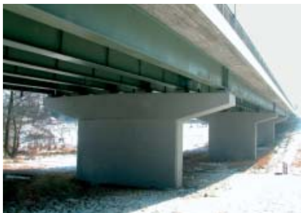
Fig. 10 By-pass between Čáslav and Golčův Jeníkov, delivery of cements Holcim (Czech Republic), JSC, member of concern
