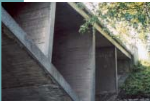
Fig. 2 View of the bridge arch, load-bearing walls and bridge deck with bare corroding reinforcement, and efflorescence of salts from percolating water
