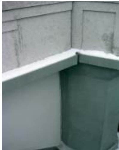
Obr. 5 ... a totéž po sanaci Fig. 5 ... and the same view after the repair completion
