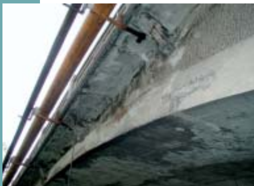
Fig. 1 Initial state – degraded cantilever with meshes
