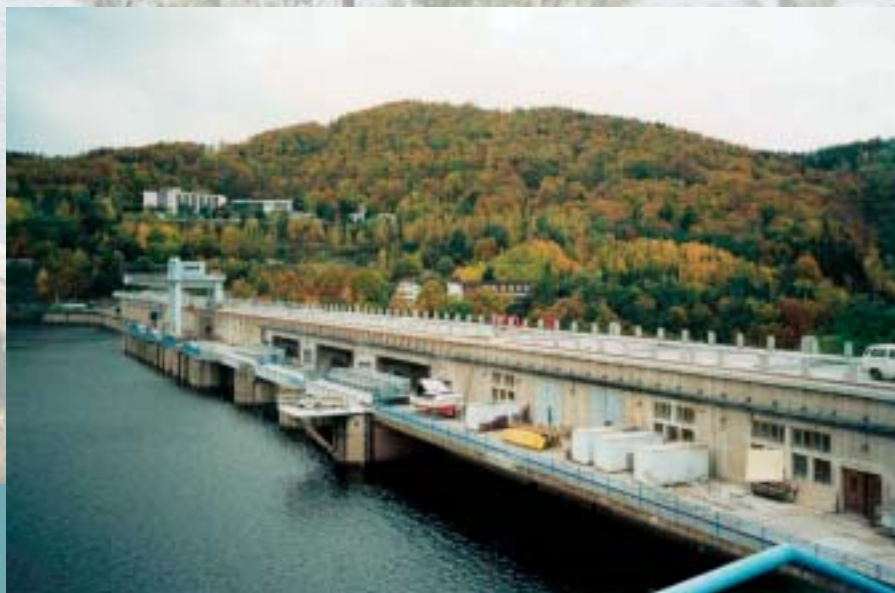
Oprava koruny hráze VD Orlík Repair of the crown of the dam of the Orlík hydraulic structure
