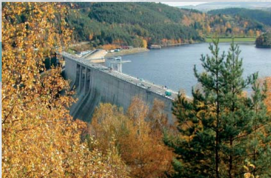
Oprava koruny hráze VD Orlík Repair of the crown of the dam of the Orlík hydraulic structure
