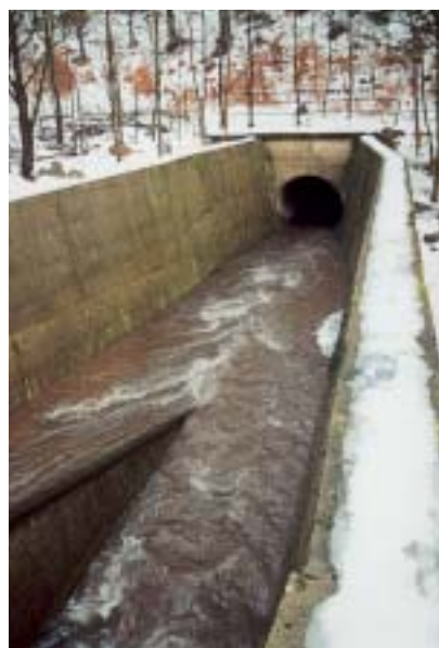
Obr. 2 Betonový žlab na vtoku do štoly Fig. 2 Concrete flume at the inlet into the tunnel
