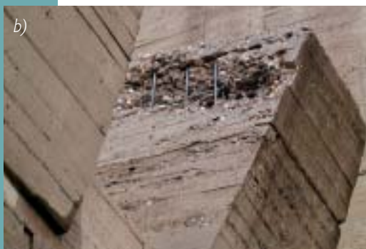
Fig. 6 Damaged baffle-blocks at the end of the overflow surface after flood; a) general view, b) detail
