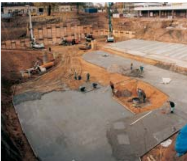
Fig. 5 Basis concrete below insulation applied on the heads of the completed piles
