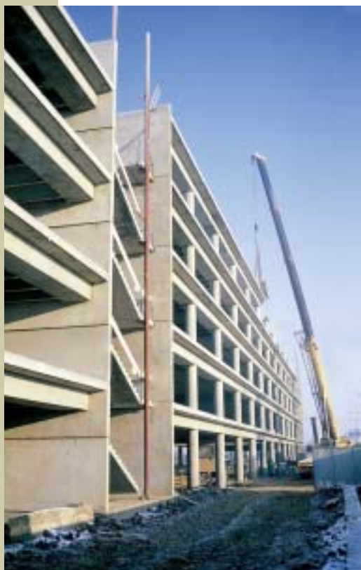
Fig. 7 Assembly of the initial section of 15.6 m along the whole height of the building
