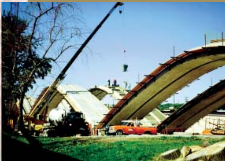
Betonáž oblouku mostu na Wisconsin Avenue, Milwaukee, Wisconsin, USA Casting of the arch of the Wisconsin Avenue Bridge, Milwaukee, Wisconsin, USA
