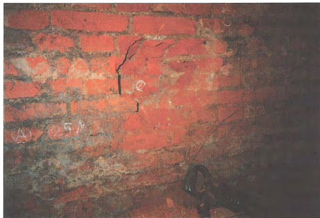
Obr. 1 – Stav cihelného zdiva v suterénu / State of the masonry on the underground floor before the repair
