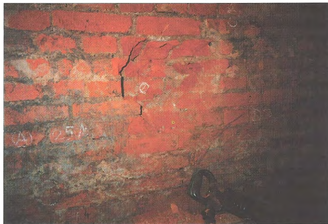
Obr. 1 – Stav cihelného zdiva v suterénu / State of the masonry on the underground floor before the repair
