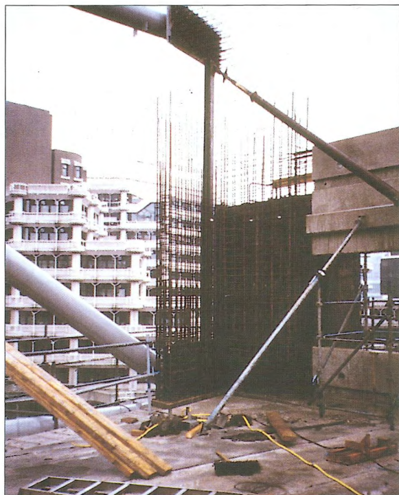
Obr. 8 – Prefabrikované betonové stropy, ocelová tuzidla a monolitické sloupy spojené v prostorovou konstrukci / Precast concrete floors, structural steel bracing and cast in situ columns integrating 2-dimensional elements into 3-dimensional structure
