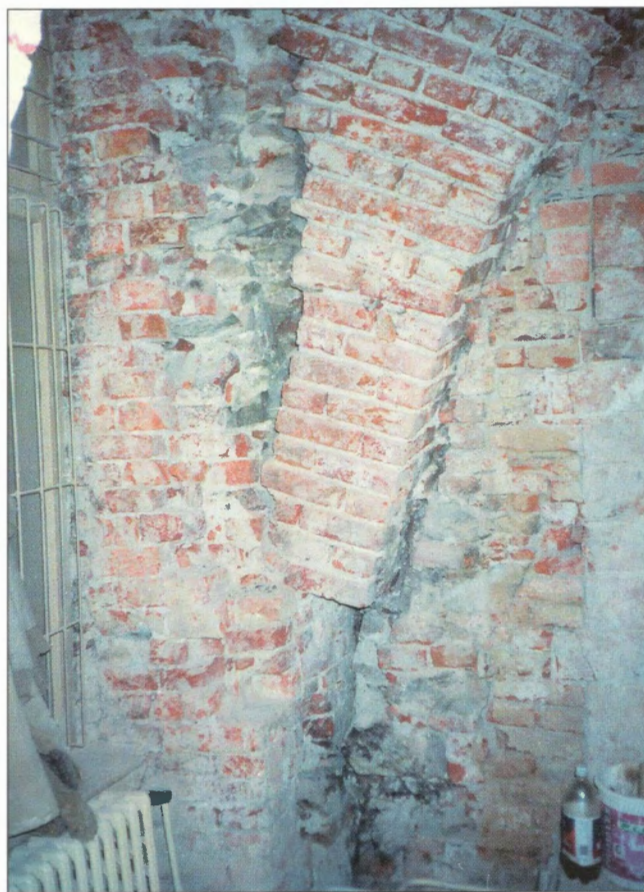
Obr. 7 – Detail trhlin a porušené paty klenby v přízemí / Detail of the cracks and damaged foot of the vault on the ground floor
